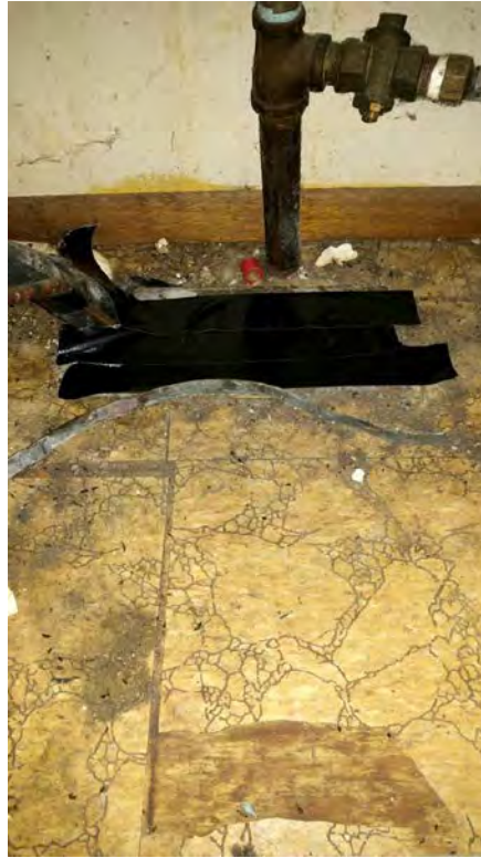
Photo of floor vent from furnace closet to crawl space (from August 2017 appointment).
