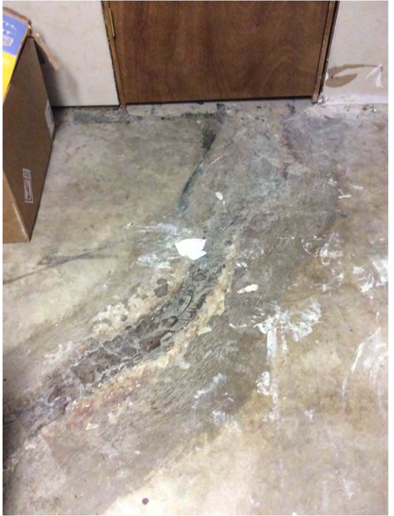
Filled crack spanning several feet from the basement door to center of room.
