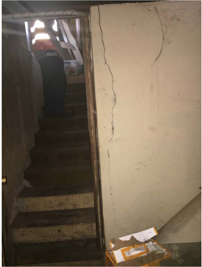
Crack located on basement wall next to garage stairwell.
