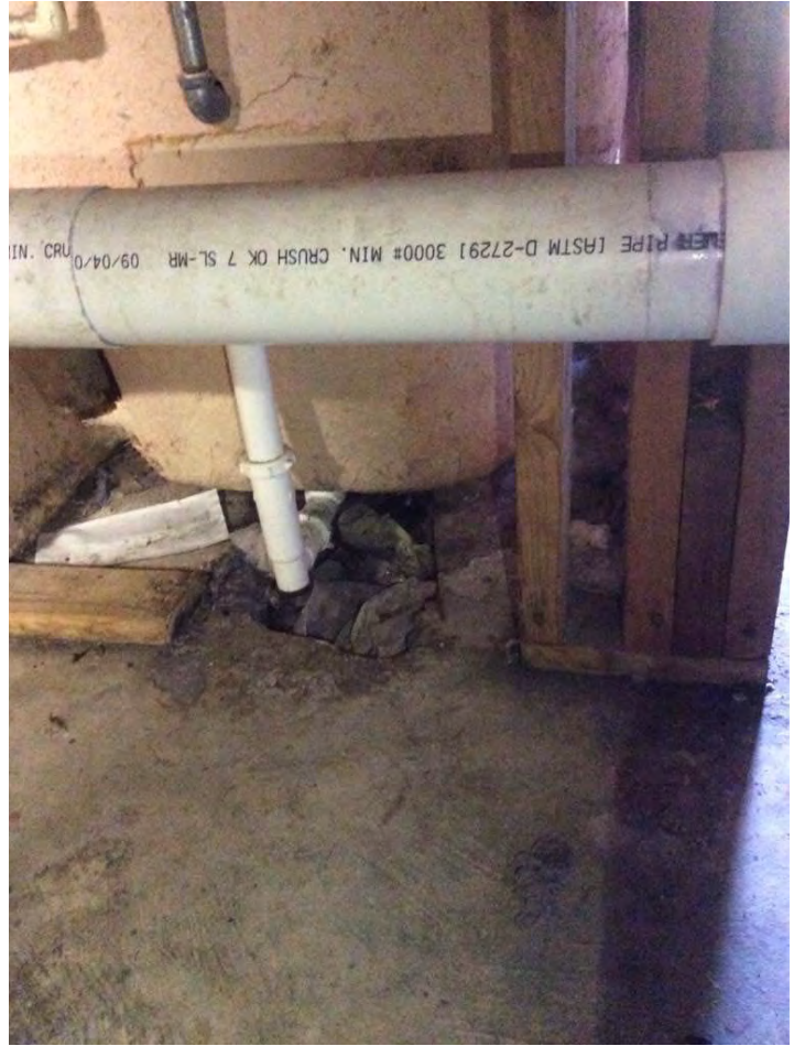
1' x 2' section of slab missing from the placement of a bathtub overflow pipe. Sub-slab is unlined and is exposed.
