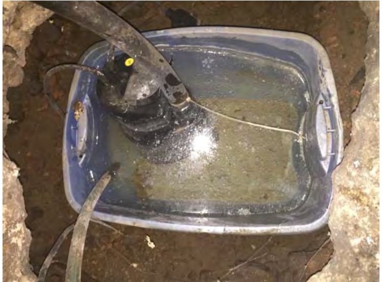
Top View of sump. Sump pump submerged in water. A dust film was observed on the surface of the water.
