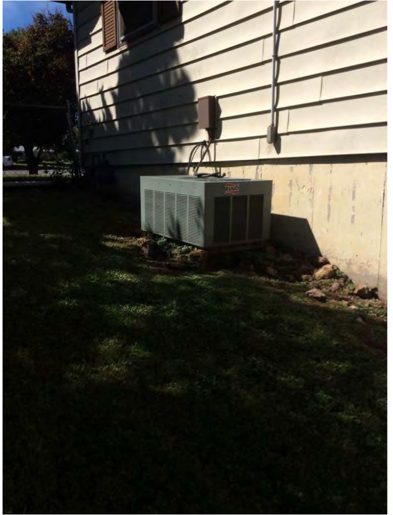
External AC unit
