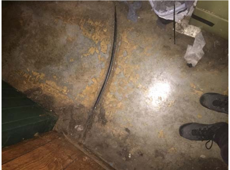
Shallow trench used for a water line runs north to south and is located near laundry hallway in basement.
