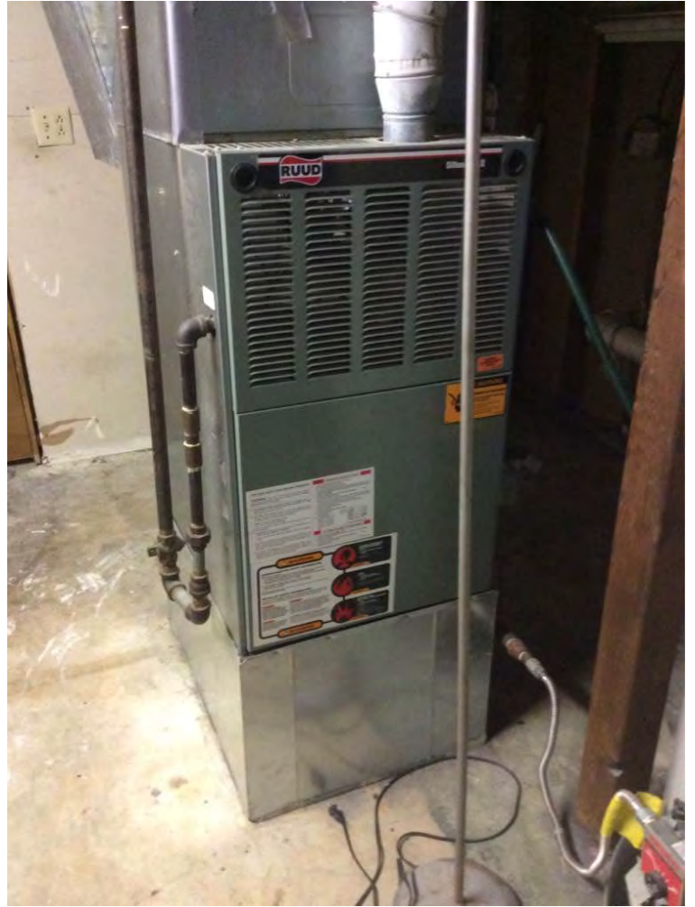
Forced hot air, natural gas furnace located in the utility room of basement.
