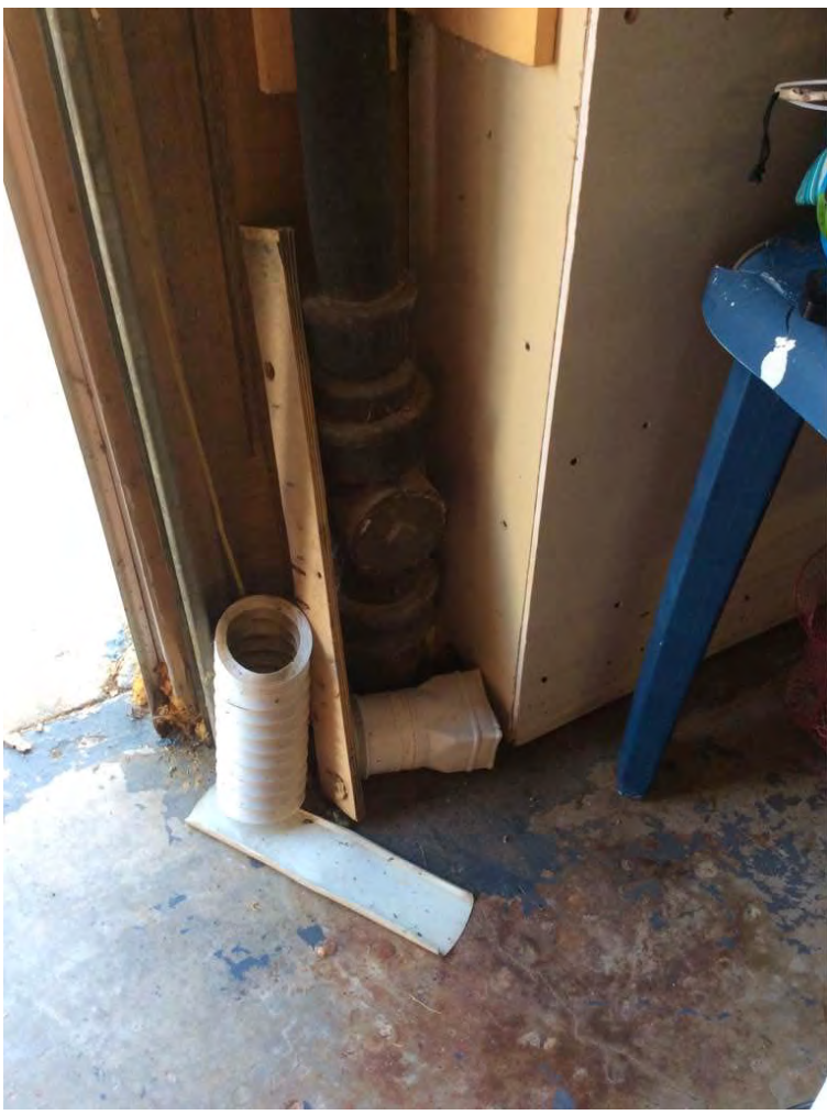
Sewer line/vent stack located in the garage by garage door.
